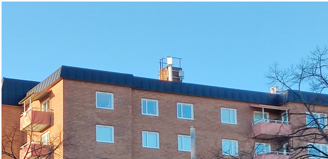
Figure 1: Top floor apartment adjacent to base stations. Two bedrooms close to the base station antennas, which are attached to the chimney.
